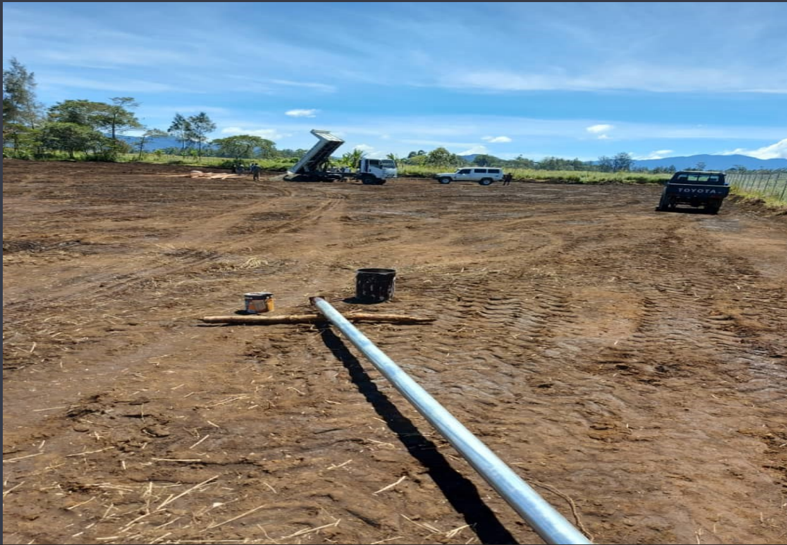
Land has been cleared and construction is now underway for the Public Services Commission's first ever Highlands regional office in Mt Hagen, Western Highlands Province. Pic courtesy of Atika Investment Ltd
